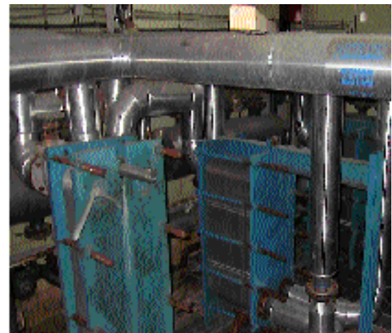
Fig.12. Characteristical parts of the "Bansko" geothermal system: Hotel "Car Samuil" (complex); Swimming pool in the hotel "Car Samuil"; Greenhouse complex (3,2 ha), and Connection station of the Hotel "Car Samuil"
