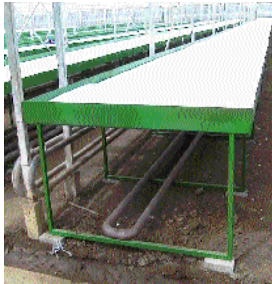
Fig.11. Geothermal heating installations in the greenhouse complex (6 ha) "Bregalnica" i Vinica
