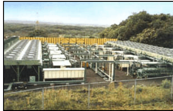
Puna Geothermal Venture, Pahoehoe, Hawaii (Photo: Ormat)
