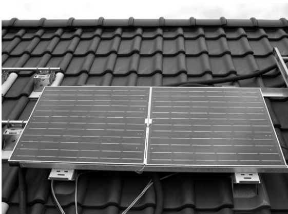
Fig. 2. Two PVT panels, installed on the PVT test facility at ECN.
