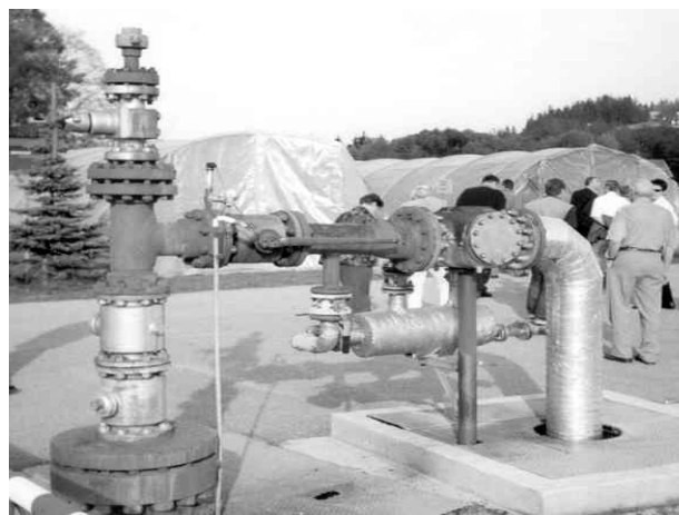
Fig. 5. Water intake (extraction well) of PASci geothermal heating plant in Bańska Niżna.
