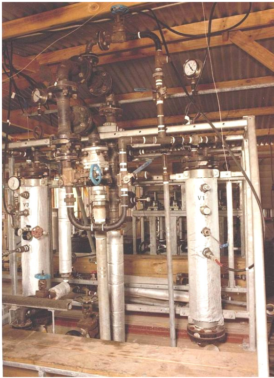
Figure 2. Test vessels for steam, V3 and two-phase fluid, V1.
